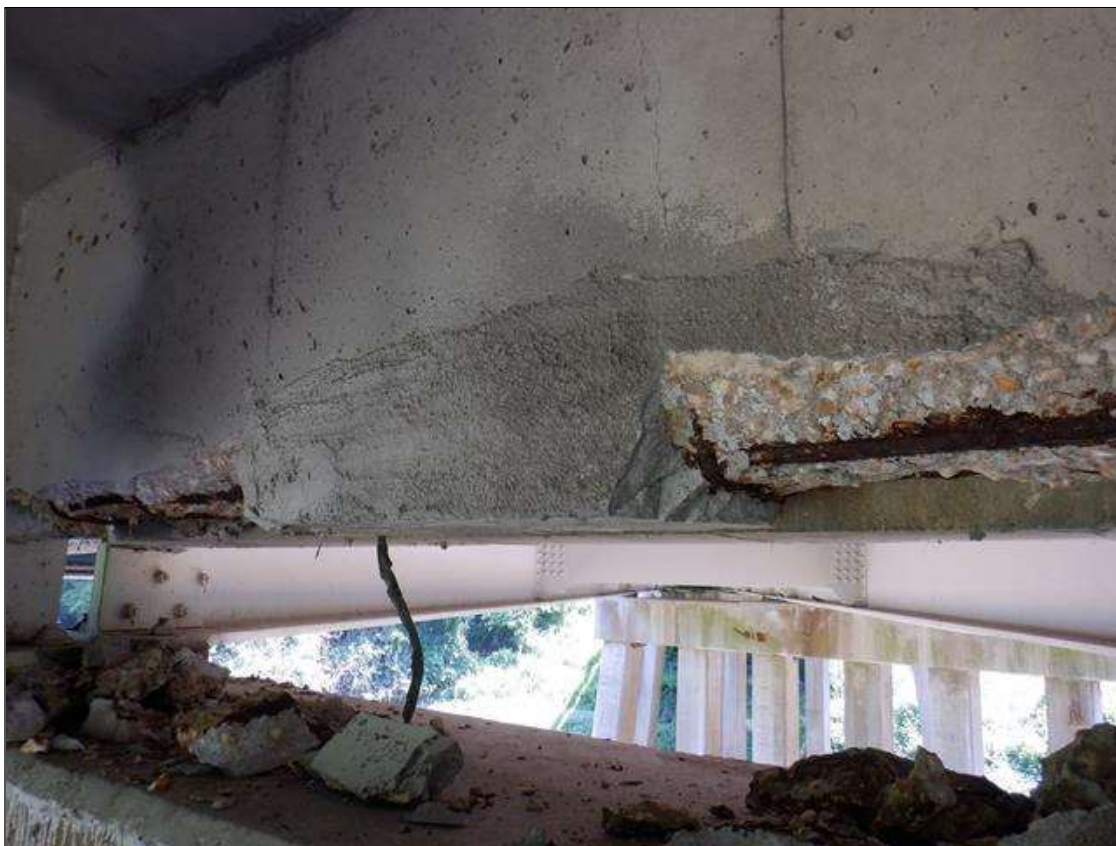
Span 4 Deck: PAR. 5 FEET LONG X 11 INCHES HIGH UNSOUND CONCRETE PATCH WITH 1/16 INCH WIDE CRACKS AND SPALLS UP TO 3 FEET X FULL WIDTH X 5 INCHES WITH EXPOSED REBAR UP TO 100 PERCENT SECTION LOSS IN BAY 1 AND EXTERIOR END DIAPHRAGM, NEXT TO BEAM 1, AT BENT 4.
