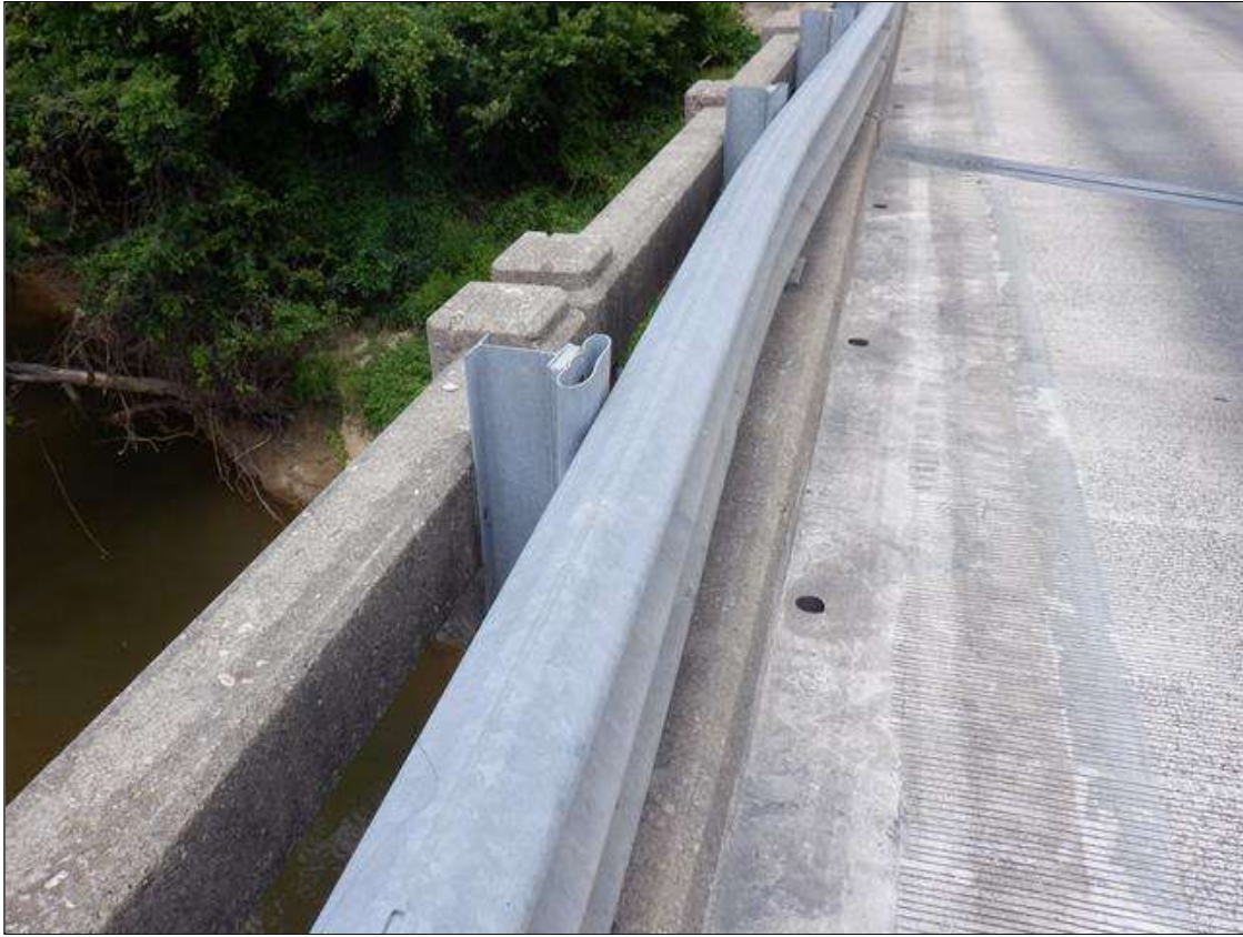
Span 6 Left Retrofit Bridge Rail: PAR, MODERATE TO HEAVY IMPACT DAMAGE WITH UP TO 5 INCHES DEFLECTION TOWARDS WEST TO THE SUPPLEMENTAL BRIDGE RAIL FOR 20 FEET LONG STARTING AT BENT 6. TWO (2) SPACER BLOCKS CONNECTING THE GUARDRAIL TO POSTS ARE PARTIALLY CRUSHED.
