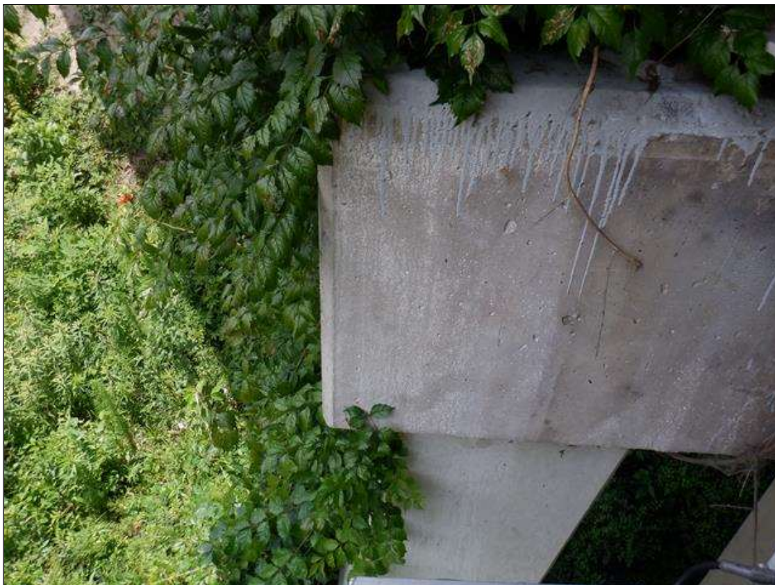
BENT 1 PILE 7 AND CAP VEGETATION GROWTH FULL HEIGHT.
