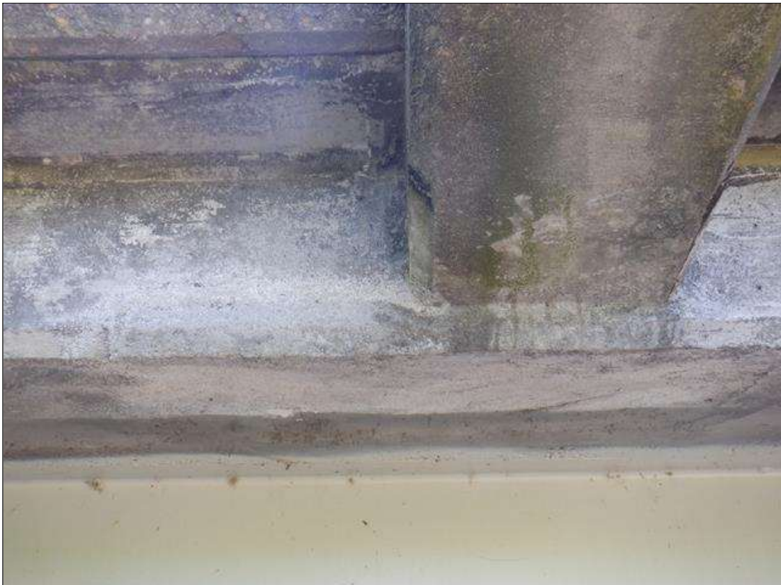
Span 7 Deck: WEST OVERHANG AT MIDSPAN 3 FEET X 15 INCHES AREA OF SOUND PATCH
