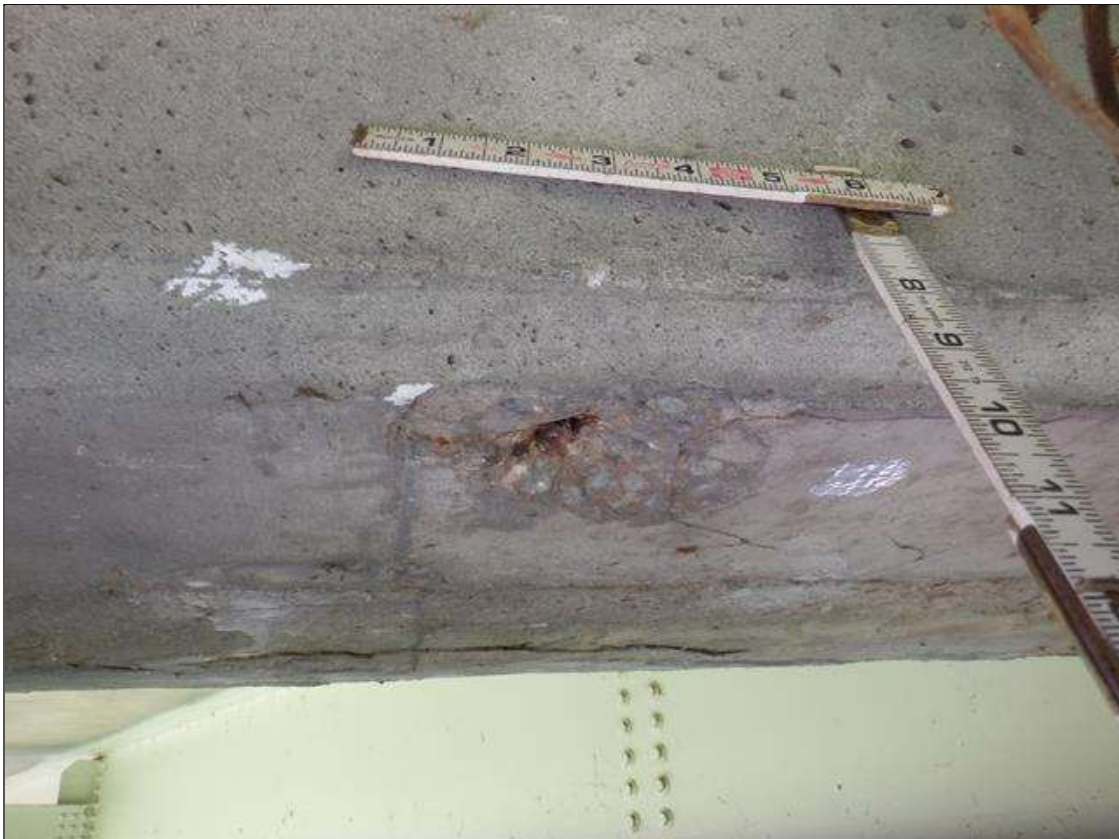
Span 2 Deck: 5 INCHES DIAMETER X 1 INCH DEEP SPALL WITH EXPOSED REINFORCEMENT IN DIAPHRAGM IN BAY 3 AT BENT 1. NO SECTION LOSS IN EXPOSED REINFORCEMENT.
