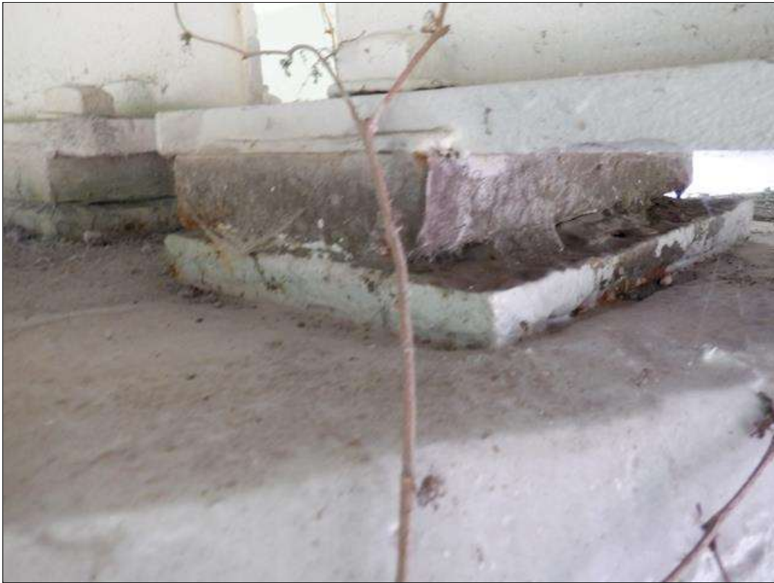
Span 7 Beam 3 - Far Bearing: SECTION LOSS REMAINS BENEATH THE PAINTED SURFACES. UP TO 90 PERCENT SECTION REMAINING IN BOTH MASONRY AND SOLE PLATES.
