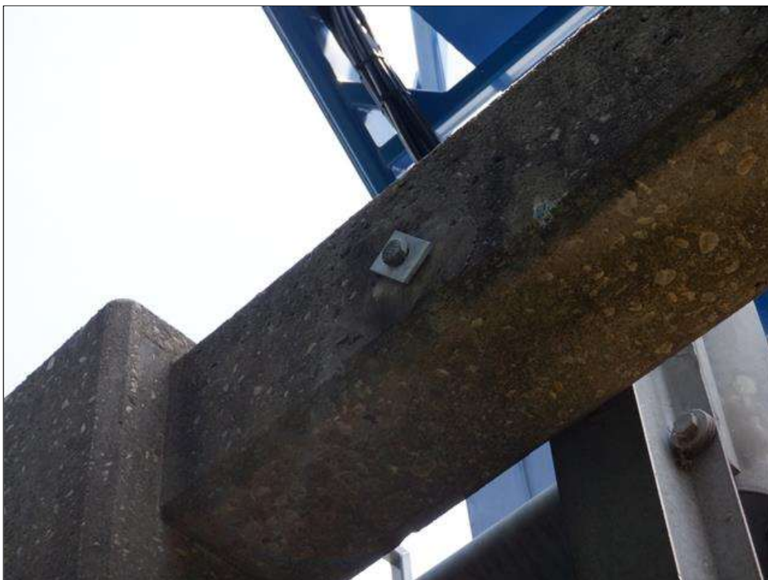
Span 1 Left Bridge Rail: 6 INCH DIAMETER SOUND PATCH AT ANCHOR BOLT CONNECTION TO RETROFIT RAIL
