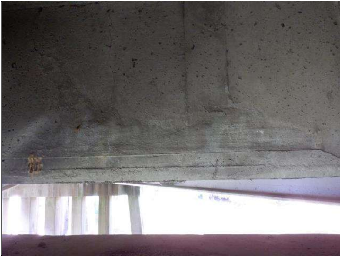
Span 8 Deck: 3 FEET LONG X 10 INCHES HIGH SOUND CONCRETE PATCHED AREA BOTTOM OF BAY 2 END DIAPHRAGM, AT BENT 7.
