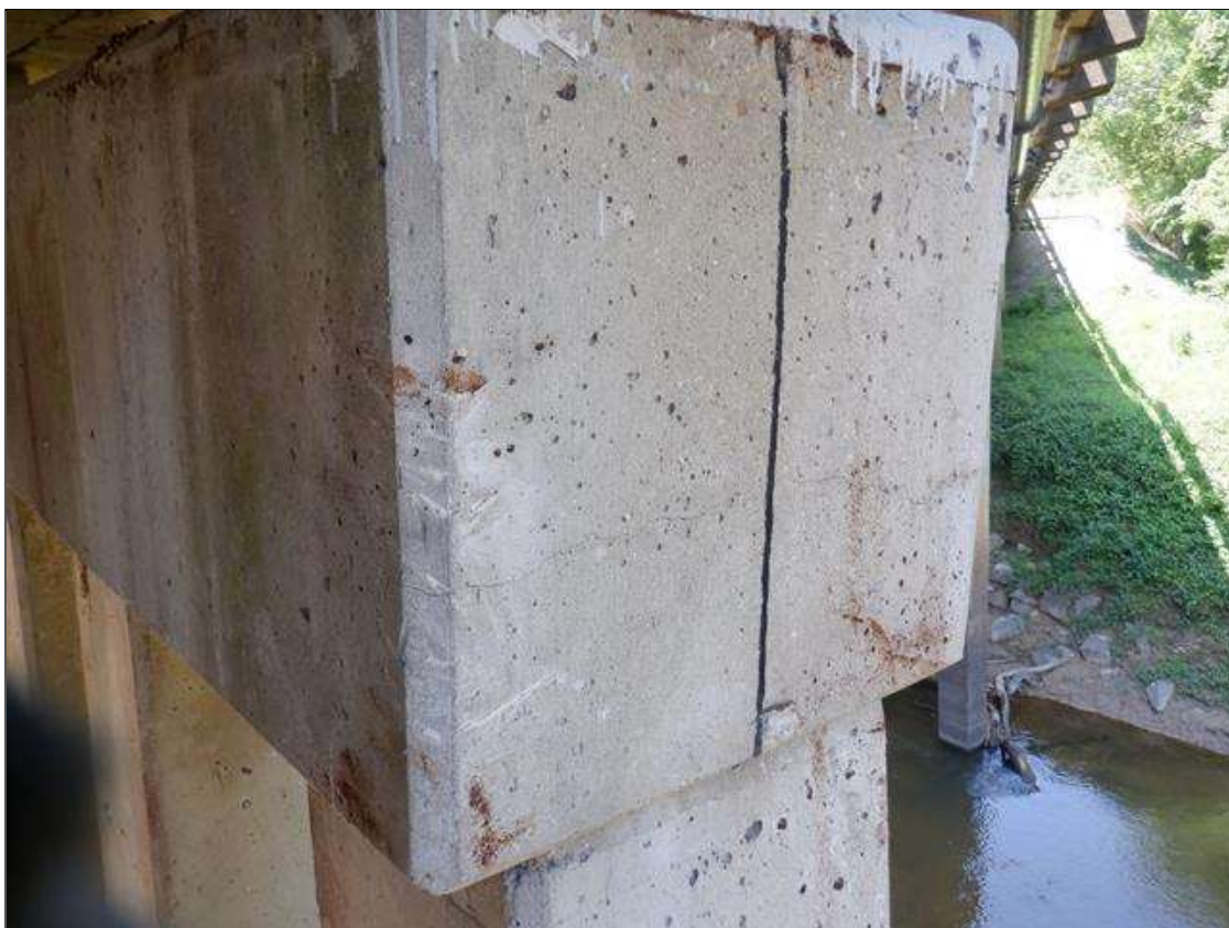
Bent 4 Cap 1: 30 INCHES LONG X 1/16 INCH WIDE HORIZONTAL CRACK, CENTER OF WEST END.
