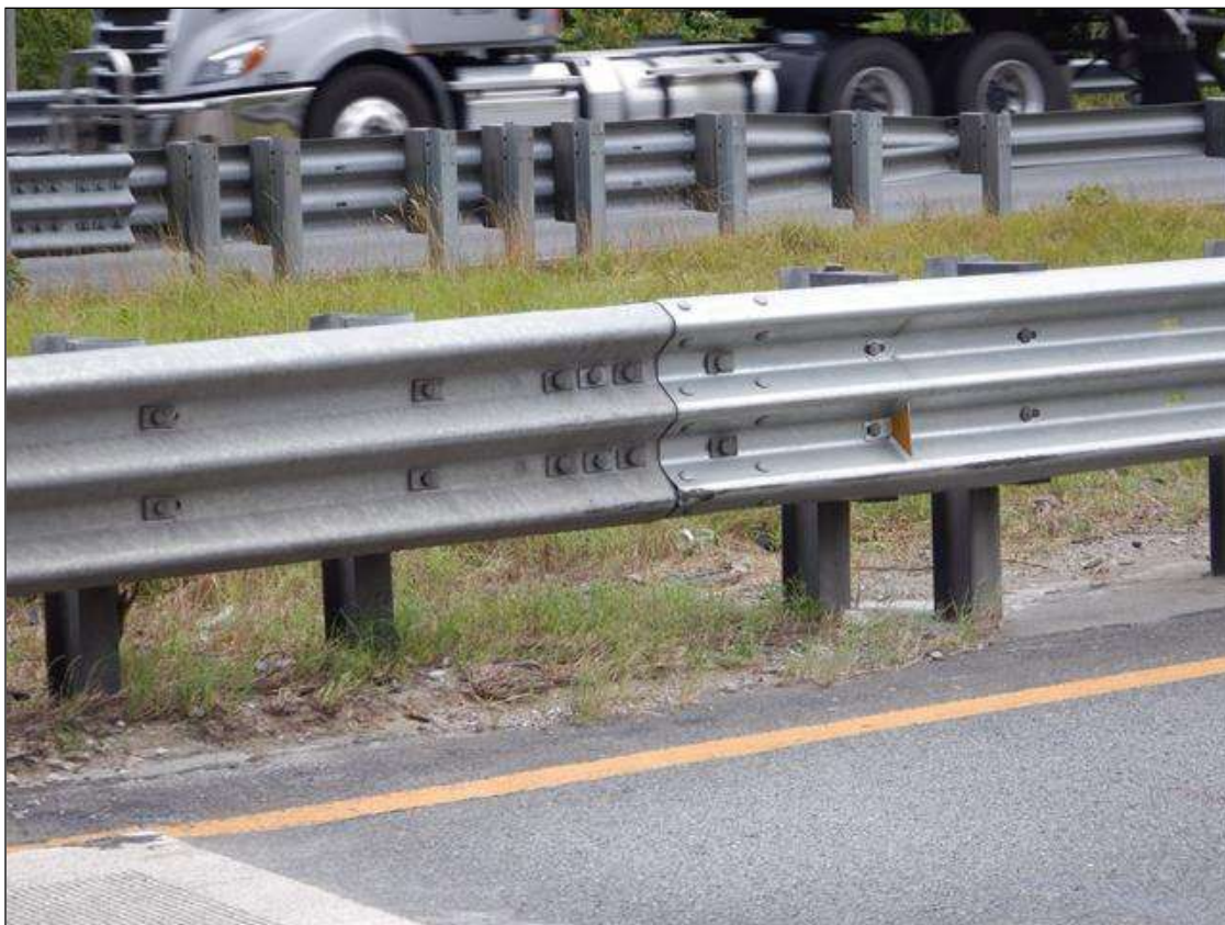
PAR. SOUTHEAST GUARDRAIL AT APPROACH LAPPED OPPOSITE TRAFFIC.
