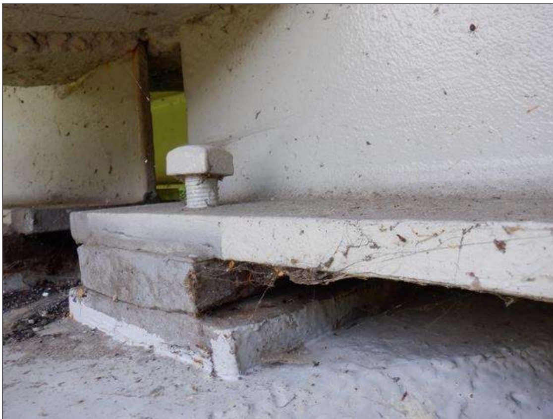
Span 3 Beam 4: PAR. RIGHT ANCHOR BOLT NUT LOOSE.
