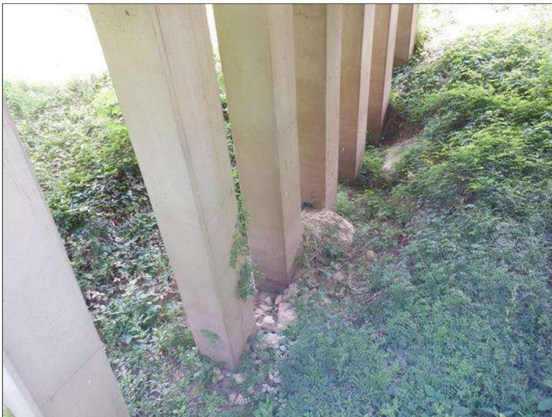
AT BENT 1 SCOUR HOLE 50 FEET X 20 FEET X 3 FEET.
