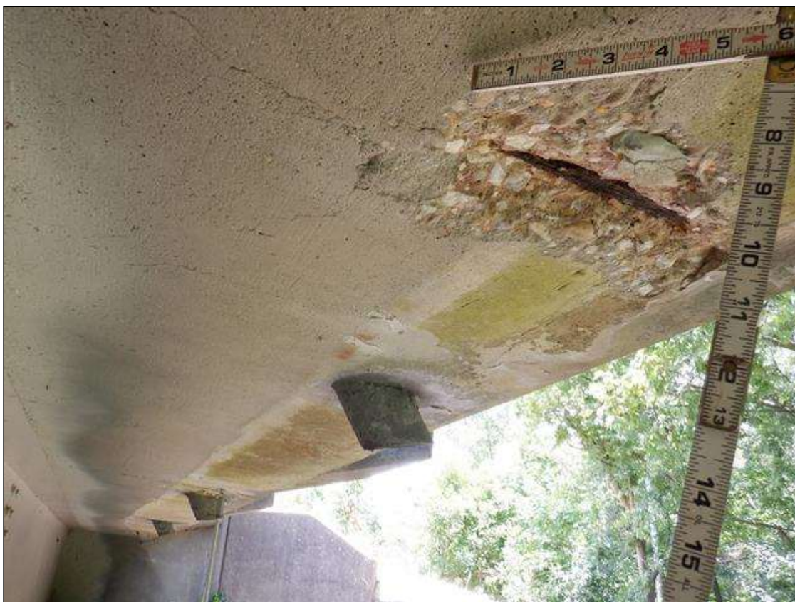
Span 1 Deck: PAR. 12 INCHES DIAMETER X 1.5 INCHES DEEP SPALL WITH EXPOSED REBAR WITH 5 PERCENT SECTION LOSS AT DRAINS 3 AND 4 IN LEFT OVERHANG.
