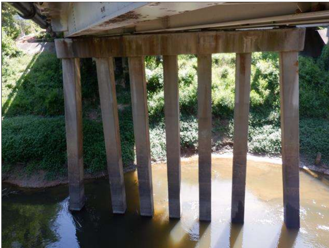
BEHIND BENT 6 AT NORTH BANK 50 FEET X 100 FEET X 6 FEET DEEP AREA OF SCOUR.
