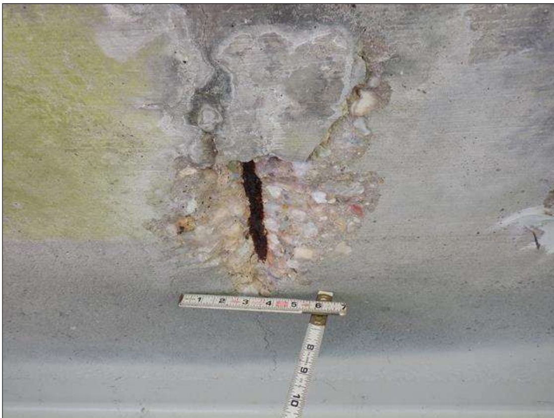
Span 2 Deck: PAR. 15 FEET FROM BENT 2 IN LEFT OVERHANG SOFFIT SPALL WITH EXPOSED REBAR 6 INCHES X 8 INCHES X 1 INCH, 5 PERCENT SECTION LOSS.
