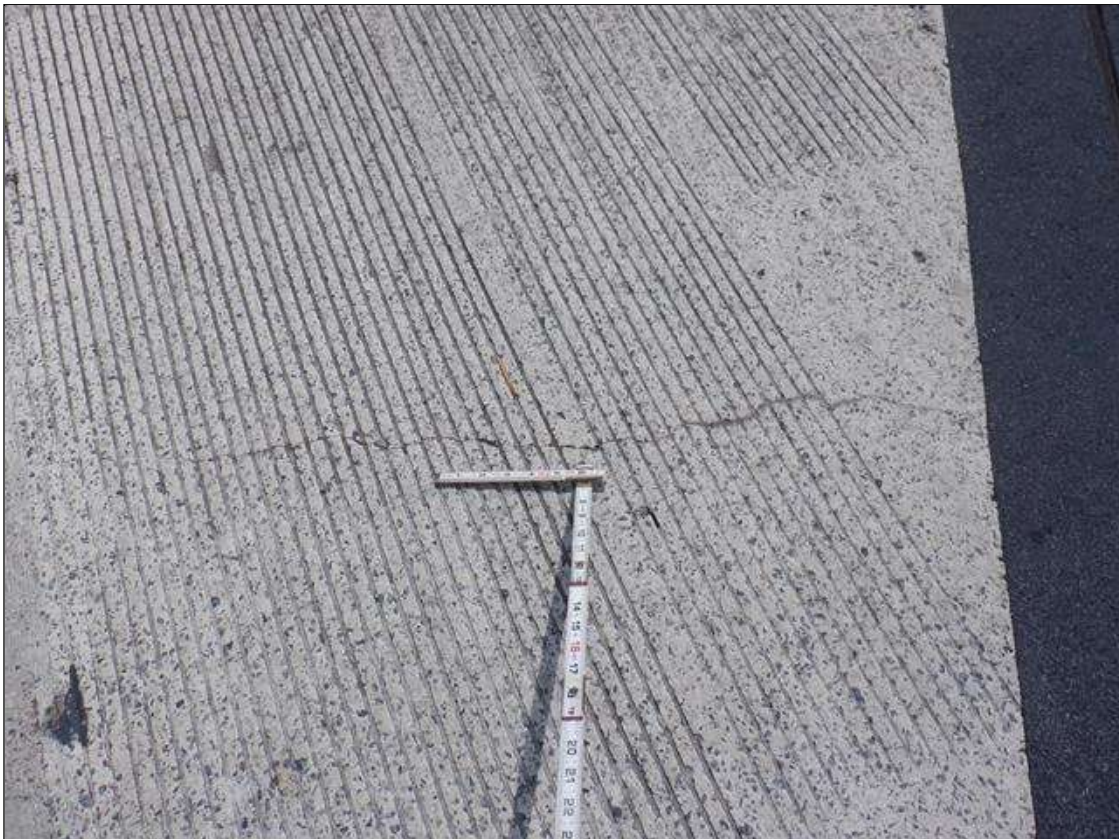
Span 1 Deck: UP TO 5 FEET LONG X 1/16 INCH WIDE LONGITUDINAL AND DIAGONAL CRACKS IN BOTH TRAVEL LANES, SCATTERED.
