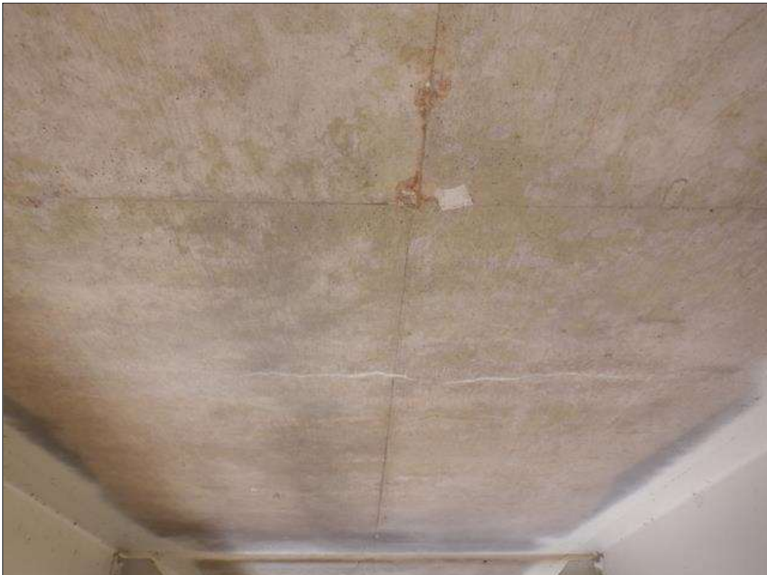
Span 5 Deck: UP TO 0.02 INCH WIDE RANDOM CRACKING IN DECK UNDERSIDE IN ALL BAYS, SOME WITH EFFLORESCENCE, SCATTERED THROUGHOUT.
