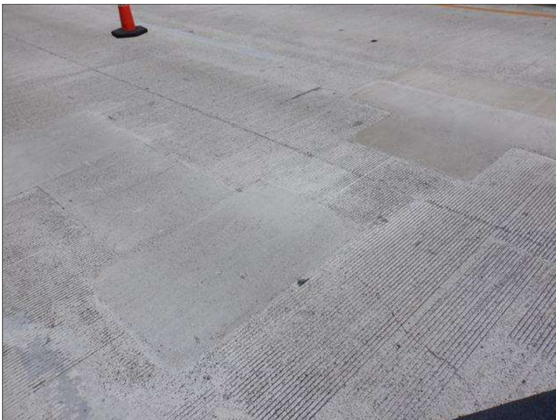
Span 1 Deck: NEAR END BENT 1 IN BOTH LANES PATCHES UP TO 6 FEET X 6 FEET
