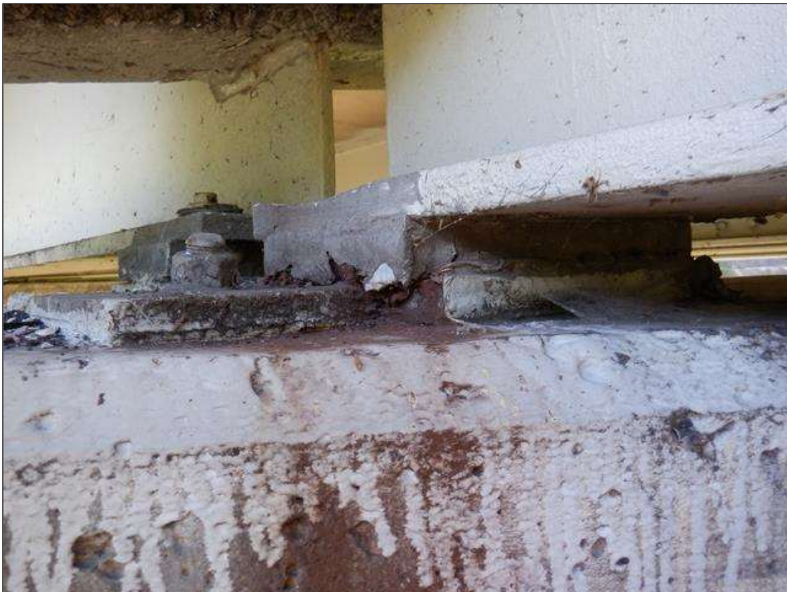
Span 6 Beam 1 - Far Bearing: BEARING ASSEMBLY HAS WELDED REPAIR WITH ADDED ANCHOR BOLT.
