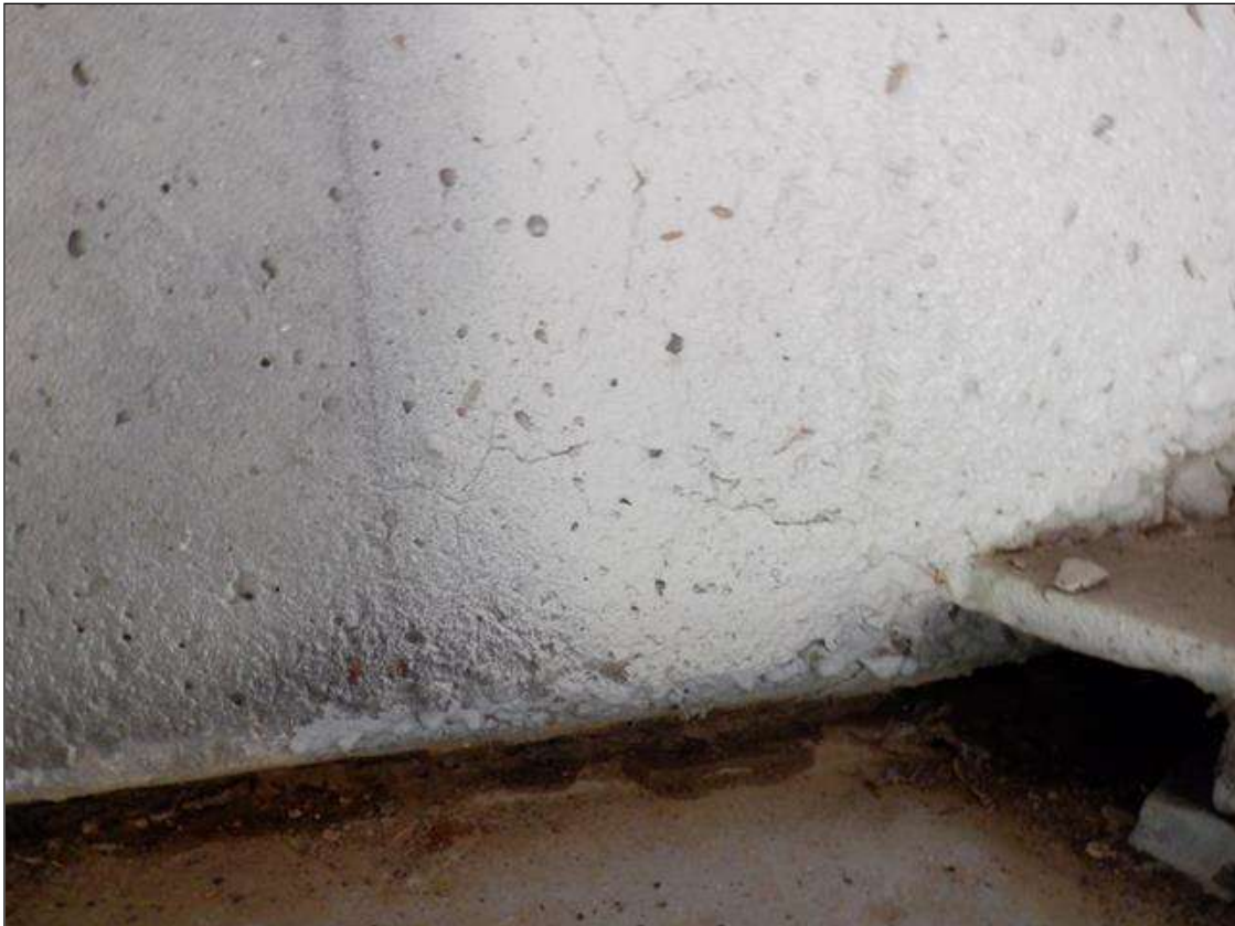
End Bent 2 Abutment: UP TO 1/16 INCH WIDE X 2 FEET LONG DIAGONAL CRACKS EXTENDING FROM BEARING AT ALL BEAMS
