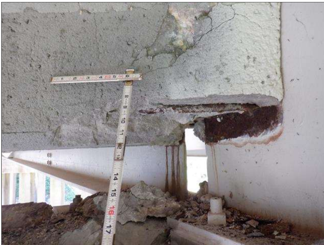
Span 7 Deck: PAR. 18 INCHES LONG X 6 INCHES HIGH X 12 INCHES WIDE SPALL WITH EXPOSED REBAR IN BAY 3 END DIAPHRAGM AT BENT 6. 10 PERCENT SECTION LOSS IN THE EXPOSED REBAR.
