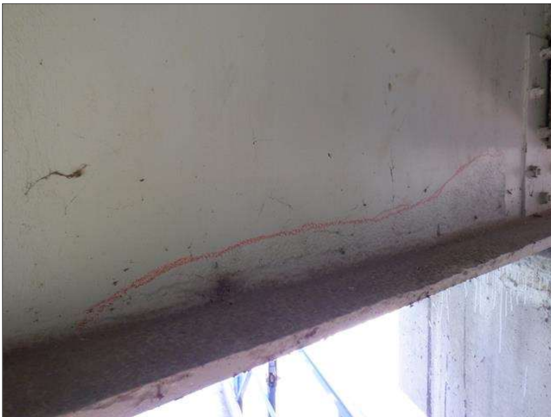
Span 3 Beam 1: 3.3 FEET LONG X UP TO 5 INCHES HIGH AREA OF RIGHT FACE OF THE WEB AT 1.25 FEET FROM BEAM END AT BENT 3 EXHIBITS SECTION LOSS BENEATH THE PAINTED SURFACE. UP TO 0.56 INCH SECTION REMAINING.
