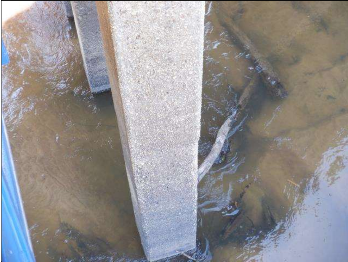
Bent 5 Pile 1: ABRASION WITH COARSE AGGREGATE EXPOSED 1/16 INCH TO 1/4 INCH LOSS OF FACIAL CONCRETE IN UPSTREAM FACE.
