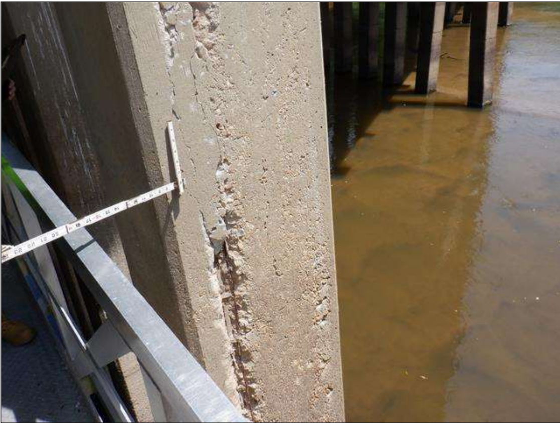
Bent 3 Pile 7: PAR. 6 FEET HIGH X 4 INCHES WIDE X 1.5 INCHES DEEP SPALL MID HEIGHT, WITH EXPOSED REINFORCEMENT IN EAST FACE. 10 PERCENT SECTION LOSS IN EXPOSED REINFORCEMENT.
