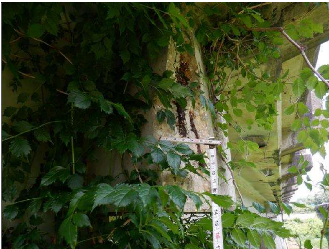
Span 1 Deck: PAR. FAR END DIAPHRAGM AT RIGHT OVERHANG SPALL WITH EXPOSED REBAR 6 INCHES X 2 FEET X 6 INCHES, 5 PERCENT SECTION LOSS.
