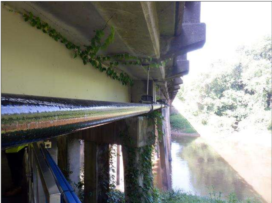
AT LEFT OVERHANG 4 INCHES DIAMETER UTILITY
