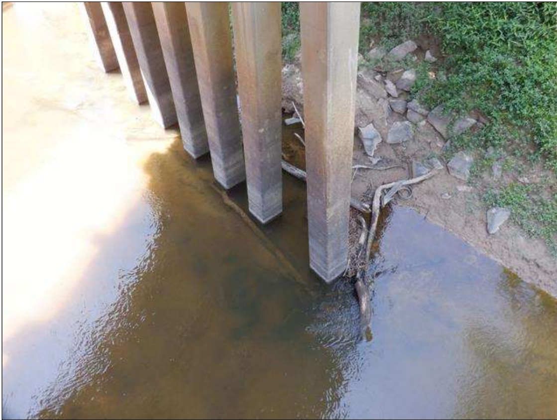
AT BENT 3 30 CUBIC FEET OF DRIFT BUILD UP.
