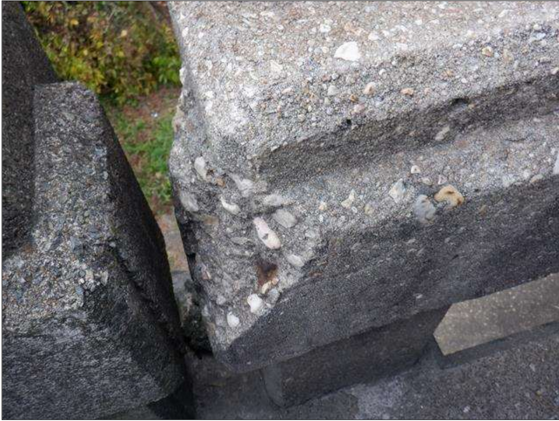
Span 8 Left Bridge Rail: TOP OF RAIL AT FIRST RAIL JOINT FROM END BENT 2, 8 INCHES WIDE X 8 INCHES HIGH X UP TO 3 INCHES DEEP SPALL WITH EXPOSED REINFORCEMENT, 10 PERCENT SECTION LOSS
