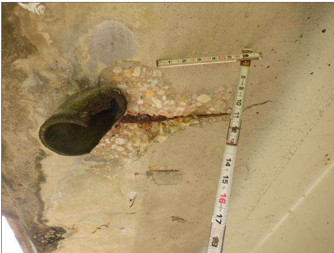
Span 1 Deck: PAR. UP TO 1 FOOT WIDE X 9 INCHES LONG X UP TO 1 INCH DEEP SPALL WITH EXPOSED REINFORCEMENT IN RIGHT OVERHANG, LOCATED AT THIRD DRAIN PIPE. 15 PERCENT SECTION LOSS IN EXPOSED REINFORCEMENT.
