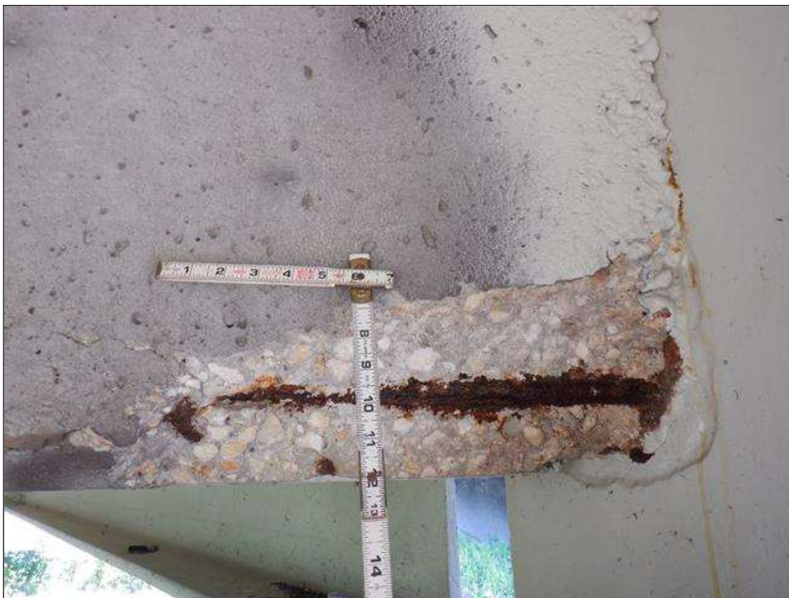
Span 6 Deck: PAR. BAY 3 FAR DIAPHRAGM ADJACENT TO BEAM 4 SPALL WITH EXPOSED REBAR 18 INCHES X 7 INCHES X 4 INCHES WITH 10 PERCENT SECTION LOSS.
