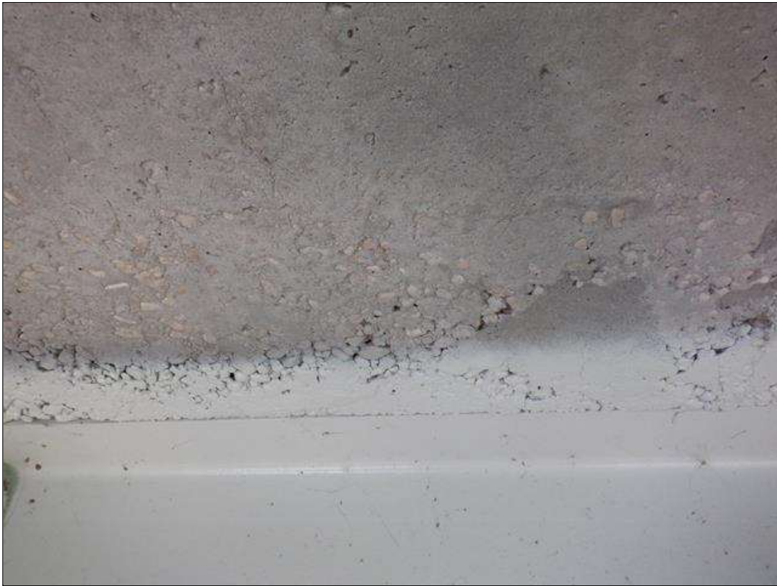
Span 7 Deck: SCATTERED AREAS OF HONEYCOMBING IN DECK UNDERSIDE IN ALL BAYS
