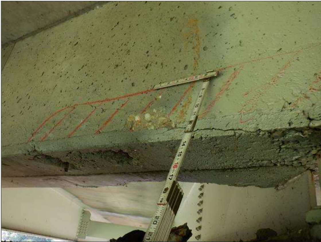
Span 2 Deck: PAR. THREE (3) 6 INCHES DIAMETER X 3/4 INCH DEEP SPALLS WITH EXPOSED REINFORCING AND AREA OF DELAMINATION 3 FEET X 7 INCHES, UNDERSIDE AND FACE OF BAY 1 END DIAPHRAGM, AT BENT 2. 10 PERCENT SECTION LOSS IN EXPOSED REINFORCEMENT.
