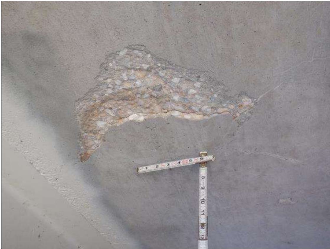
Span 6 Deck: BAY 1 NEAR BENT 6 AREA OF SPALLING 18 INCHES DIAMETER X 1/2 INCH DEEP.
