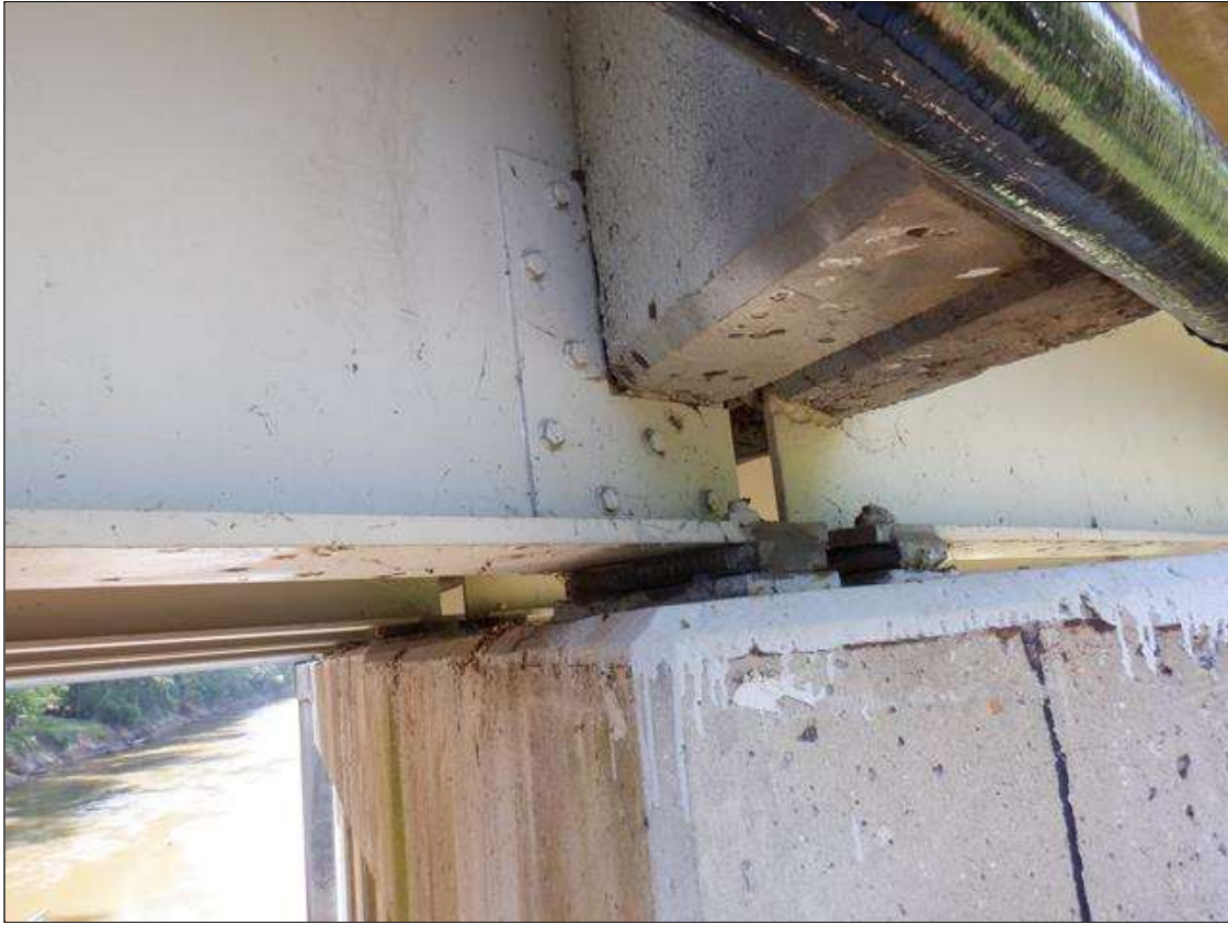
SPAN 5 BEAM 1 AT BENT 4 BOLTED PLATES ON BOTH SIDES OF WEB 20 INCHES X 16 INCHES. SIMILAR AT SPANS 2 AND 3 BEAM 1 FAR END.
