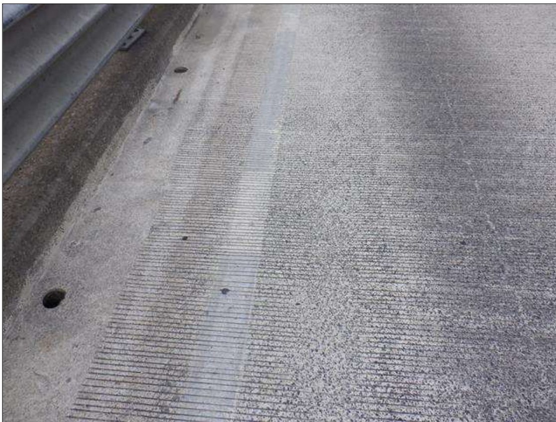
Span 4 Deck: MINOR ABRASION ON WALL MOUNT AND DECK WORN OUT WITH EXPOSED AGGREGATE IN WHEEL PATHS OF BOTH TRAVEL LANES
