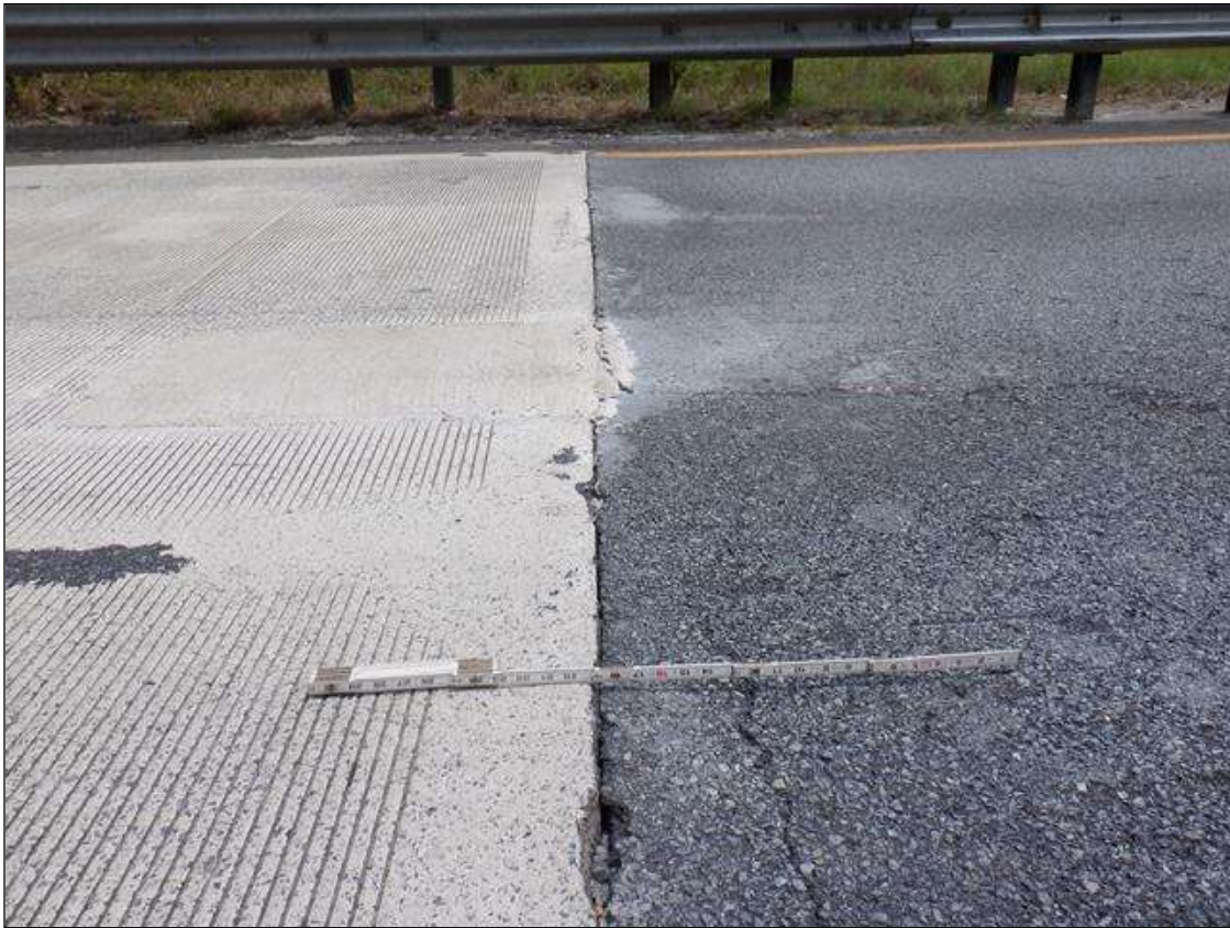
Approach 2: ASPHALT AT SOUTH END SETTLED FULL WIDTH X UP TO 1 1/2 INCH
