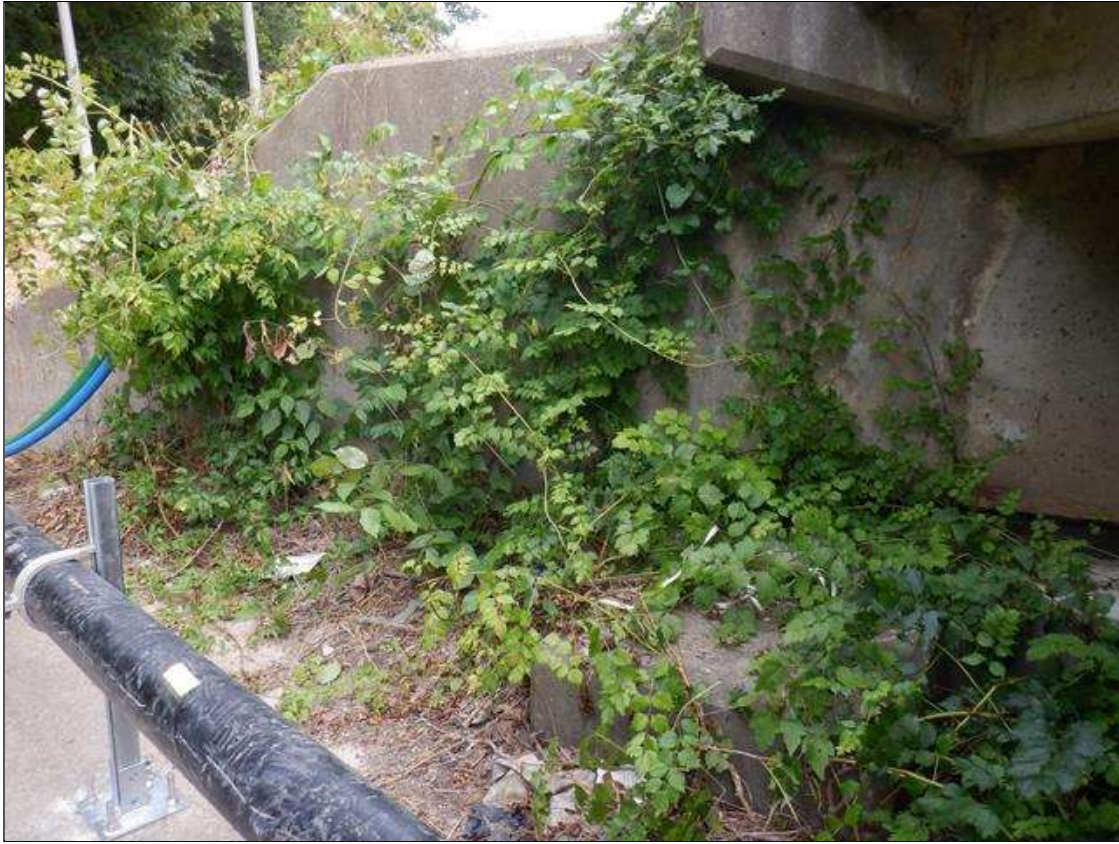
NORTHWEST WING HAS VEGETATION GROWTH. SIMILAR AT NORTHEAST.
