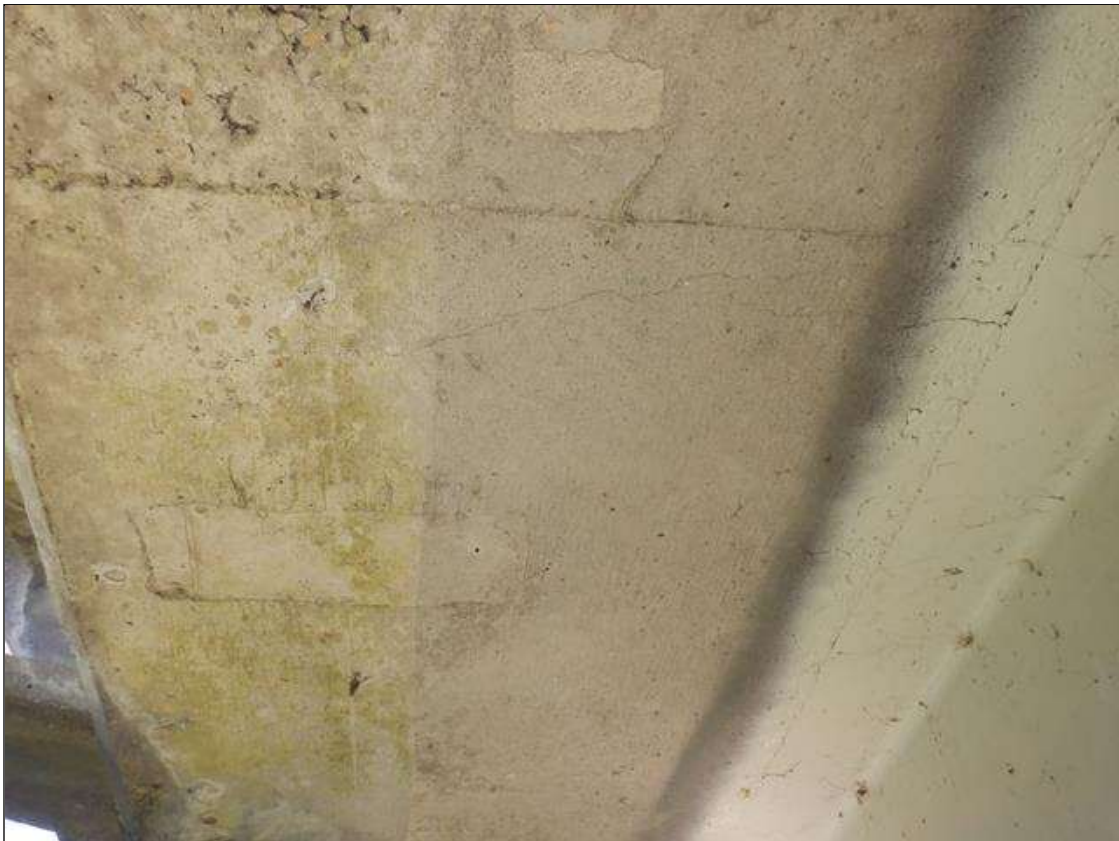
Span 7 Deck: EIGHT (8) UP TO 0.03 INCH WIDE X UP TO 3 FEET LONG TRANSVERSE CRACKS IN LEFT OVERHANG. RIGHT OVERHANG TYPICAL.
