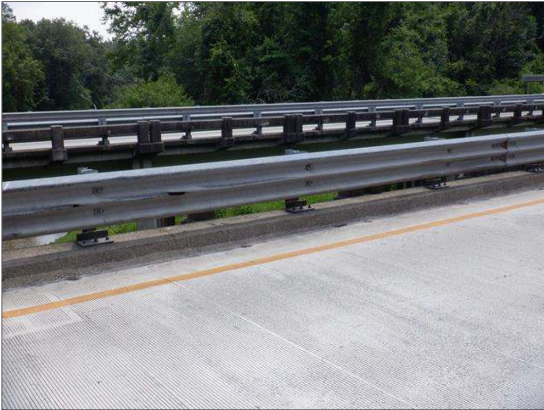
Span 2 Right Retrofit Bridge Rail: HEAVY IMPACT DAMAGE WITH SCRAPE MARKS AND THROUGH HOLES IN RETROFIT RAIL AT SCATTERED LOCATIONS
