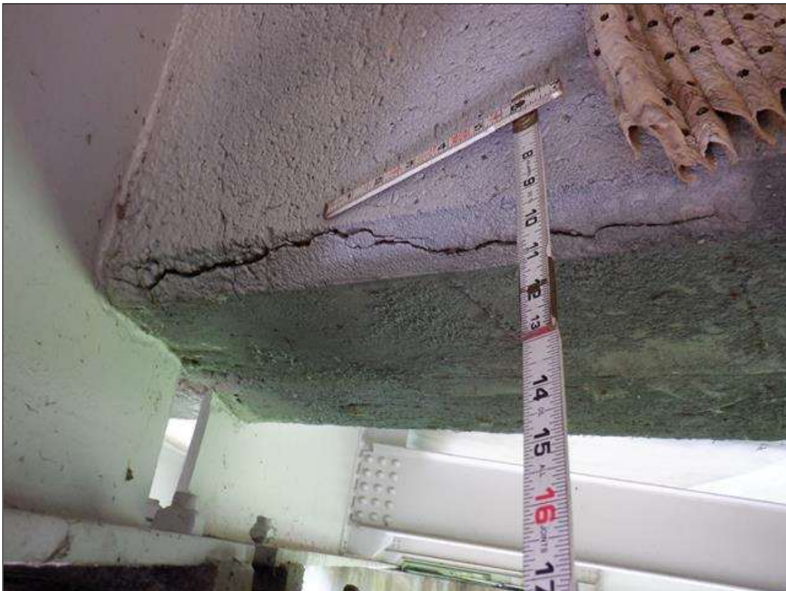
Span 4 Deck: BAY 2 NEAR DIAPHRAGM ADJACENT TO BEAM 3 AREA OF DELAMINATION 2 FEET X FULL WIDTH WITH 3/16 INCH CRACK.
