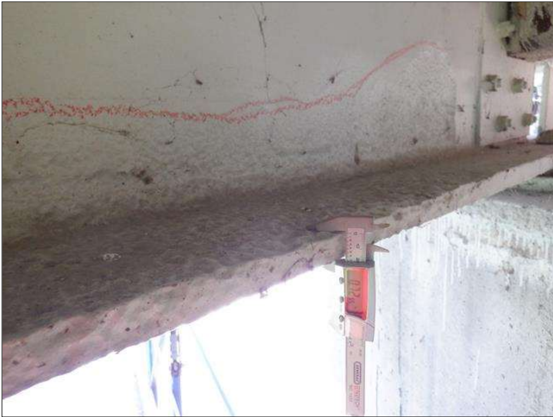
Span 3 Beam 1: 2 FEET LONG X 5 INCHES WIDE AREA OF BOTTOM FLANGE HAS SECTION LOSS BENEATH THE PAINTED SURFACE, LOCATED AT 2 FEET FROM BEAM END AT BENT 3. 0.72 INCH SECTION REMAINING.
