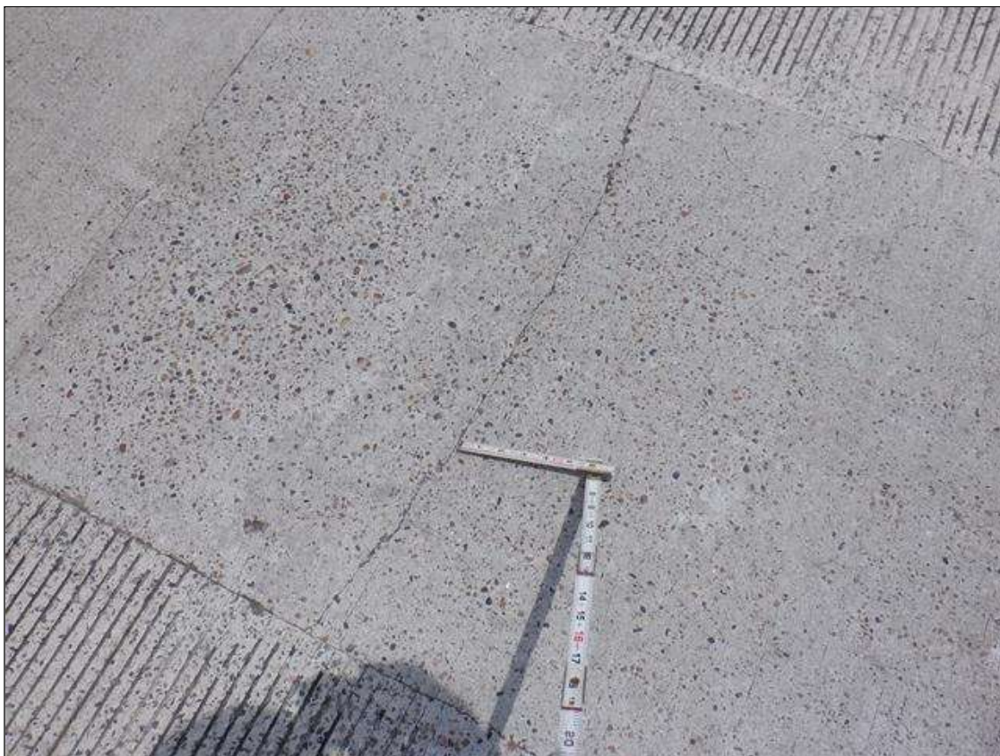
Span 1 Deck: 4 FEET LONG X 3 FEET WIDE UNSOUND CONCRETE PATCH WITH 1/16 INCH WIDE X 3 FEET LONG CRACKS EXTENDING FROM THIS PATCH IN RIGHT LANE AT END BENT 1
