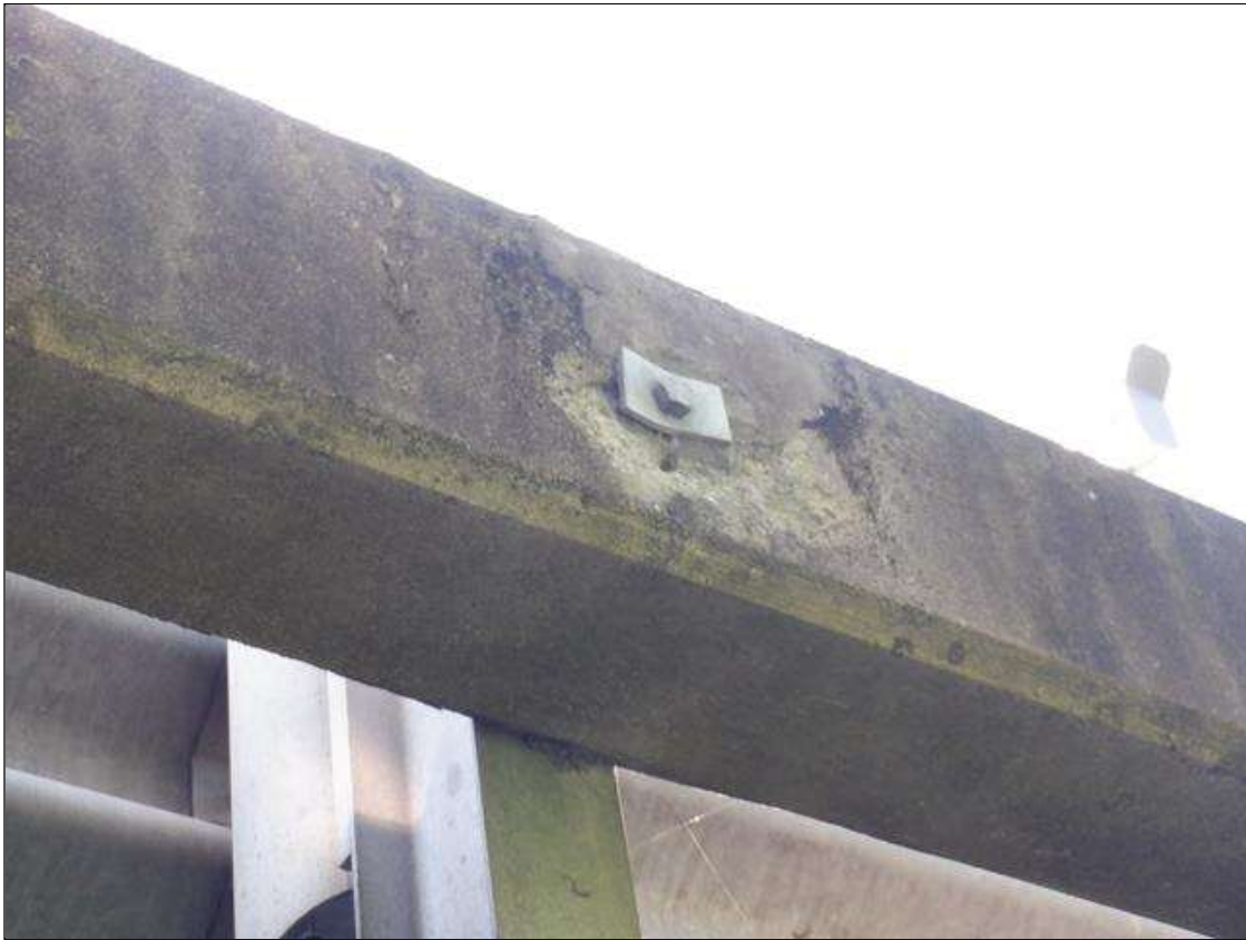
Span 8 Left Retrofit Bridge Rail: AT SECOND POST FROM END BENT 2, 6 INCH DIAMETER X 1.5 INCH DEEP SPALLS IN EXTERIOR FACE AT ANCHOR BOLT CONNECTION TO RETROFIT RAIL
