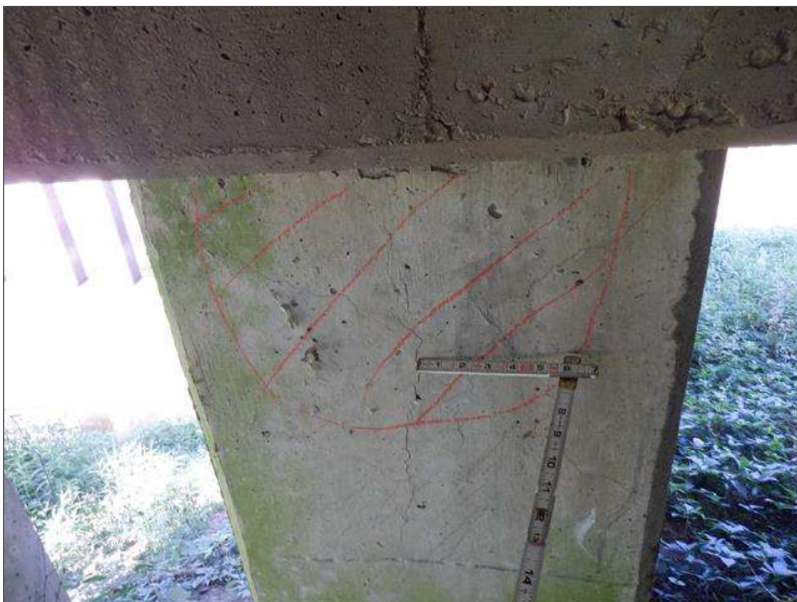
Bent 7 Pile 4: NORTH FACE UNDER CAP AREA OF DELAMINATION AND HAIRLINE CRACKING 16 INCHES DIAMETER
