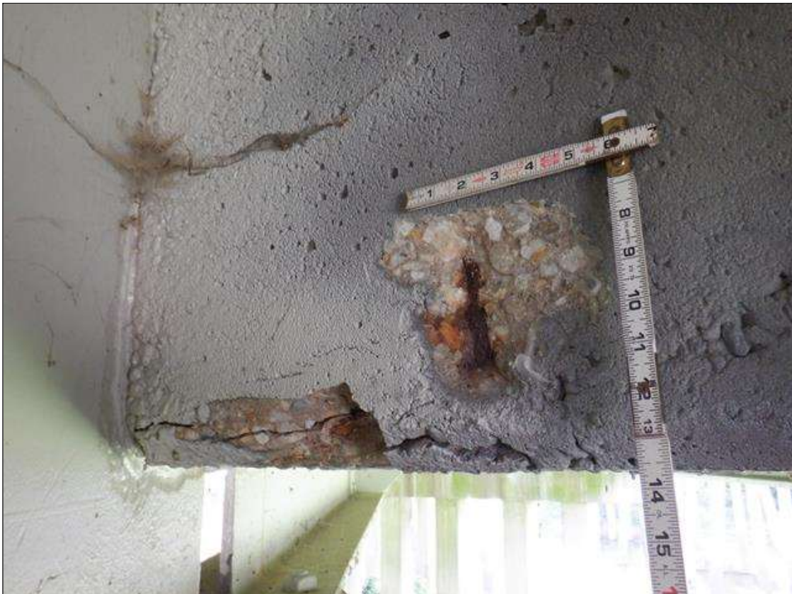
Span 1 Deck: PAR. BAY 2 FAR DIAPHRAGM ADJACENT TO BEAM 2 AREA OF DELAMINATION AND SPALLING WITH EXPOSED REBAR 1.5 FEET X 8 INCHES X UP TO 3 INCHES. 5 PERCENT SECTION LOSS.
