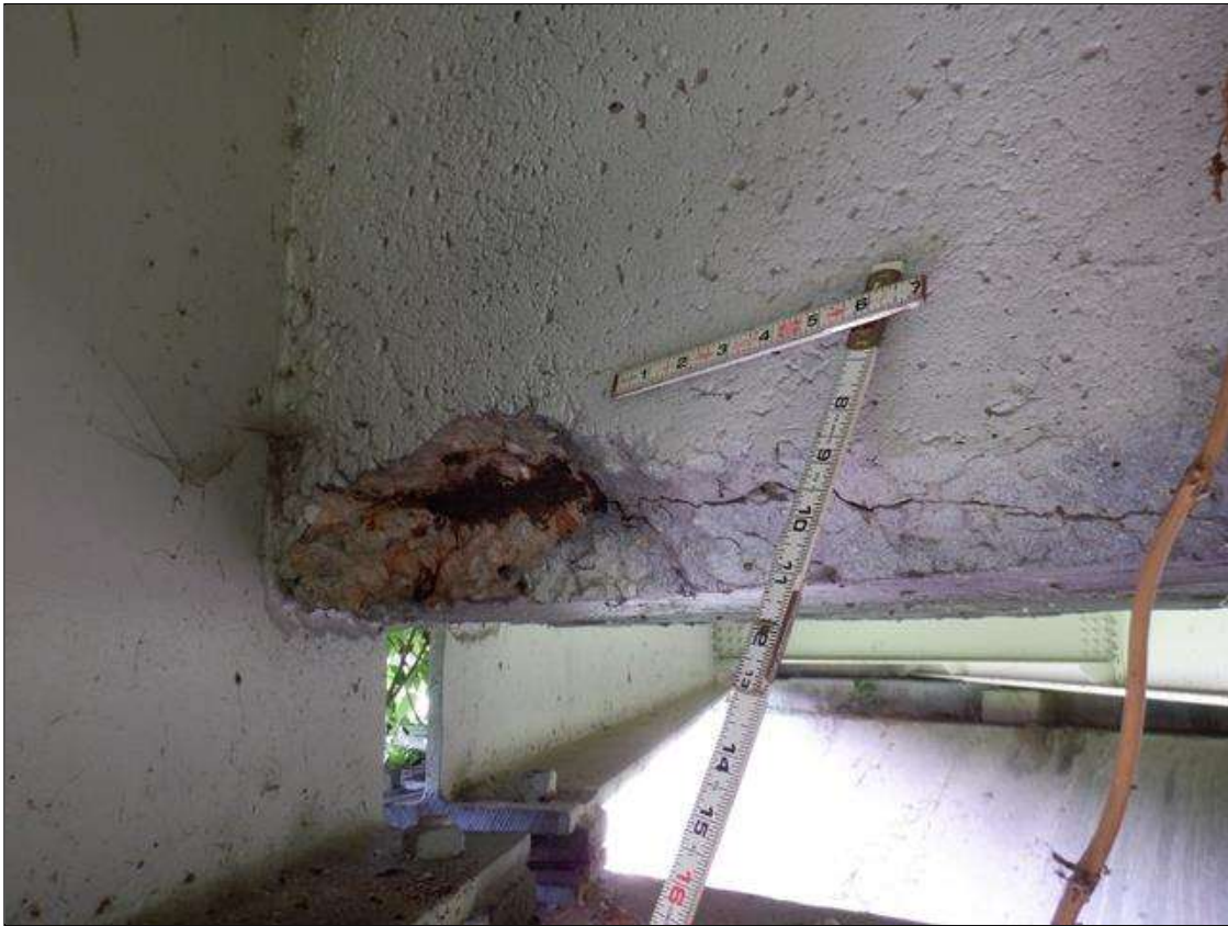
Span 2 Deck: PAR. UP TO 1.5 FEET WIDE X 4 INCHES LONG X UP TO 4 INCHES DEEP SPALL WITH EXPOSED REBAR, 5 PERCENT SECTION LOSS IN DIAPHRAGM IN BAY 3 AT BENT 1.
