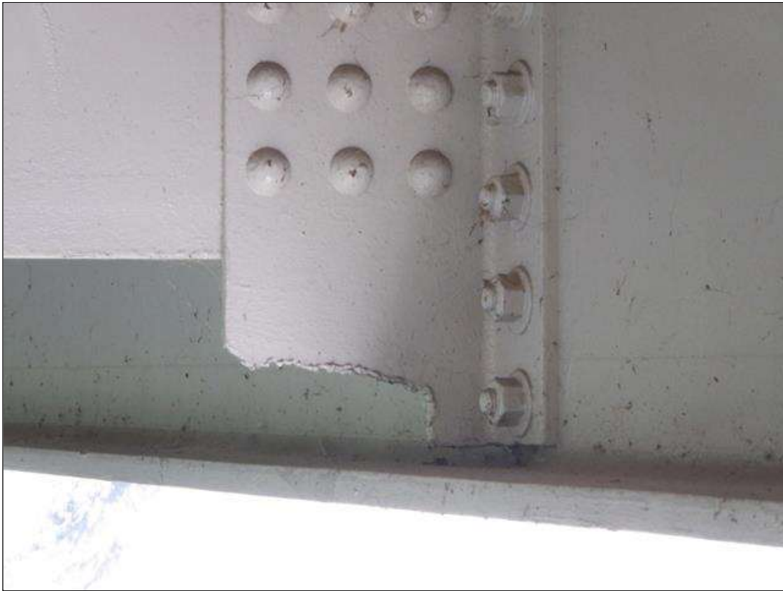
Span 7 Beam 4: UP TO 2 INCHES HIGH OF SECTION CUT OUT AT BOTTOM OF INTERMEDIATE STIFFENER. PAR IS NOT ISSUED AS IT APPEARS TO BE BRIDGE REPAIR
