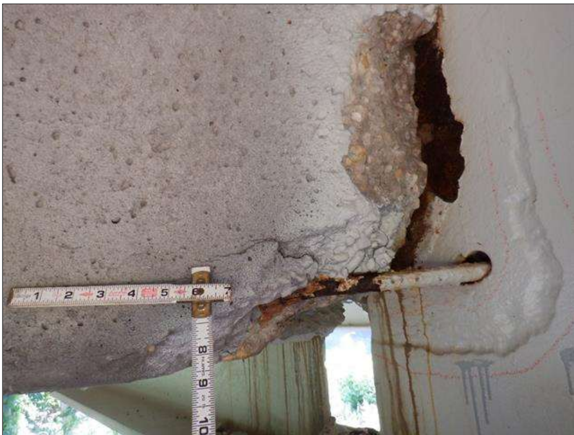
Span 6 Deck: PAR. 12 INCHES WIDE X 9 INCHES LONG X 14 INCHES HIGH SPALL IN SOUTH FACE WITH EXPOSED REINFORCEMENT IN BAY 2 AT BENT 6. 10 PERCENT SECTION LOSS IN EXPOSED REINFORCEMENT.
