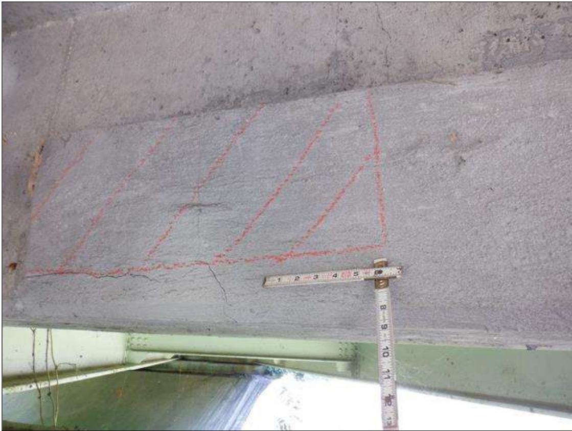
Span 7 Deck: AT BENT 7 BAY 3 DIAPHRAGM UNSOUND PATCH 7 FEET X 1 FOOT WITH 3 SQUARE FEET AREA OF DELAMINATION
