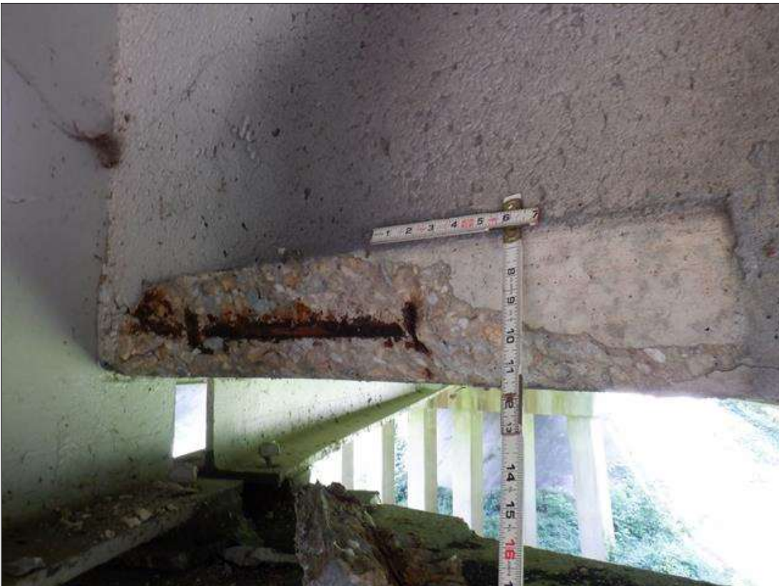
Span 3 Deck: PAR. BAY 1 NEAR DIAPHRAGM ADJACENT TO BEAM 2, SPALL WITH EXPOSED REBAR 3 FEET X 5 INCHES X 5 INCHES, 5 PERCENT SECTION LOSS.
