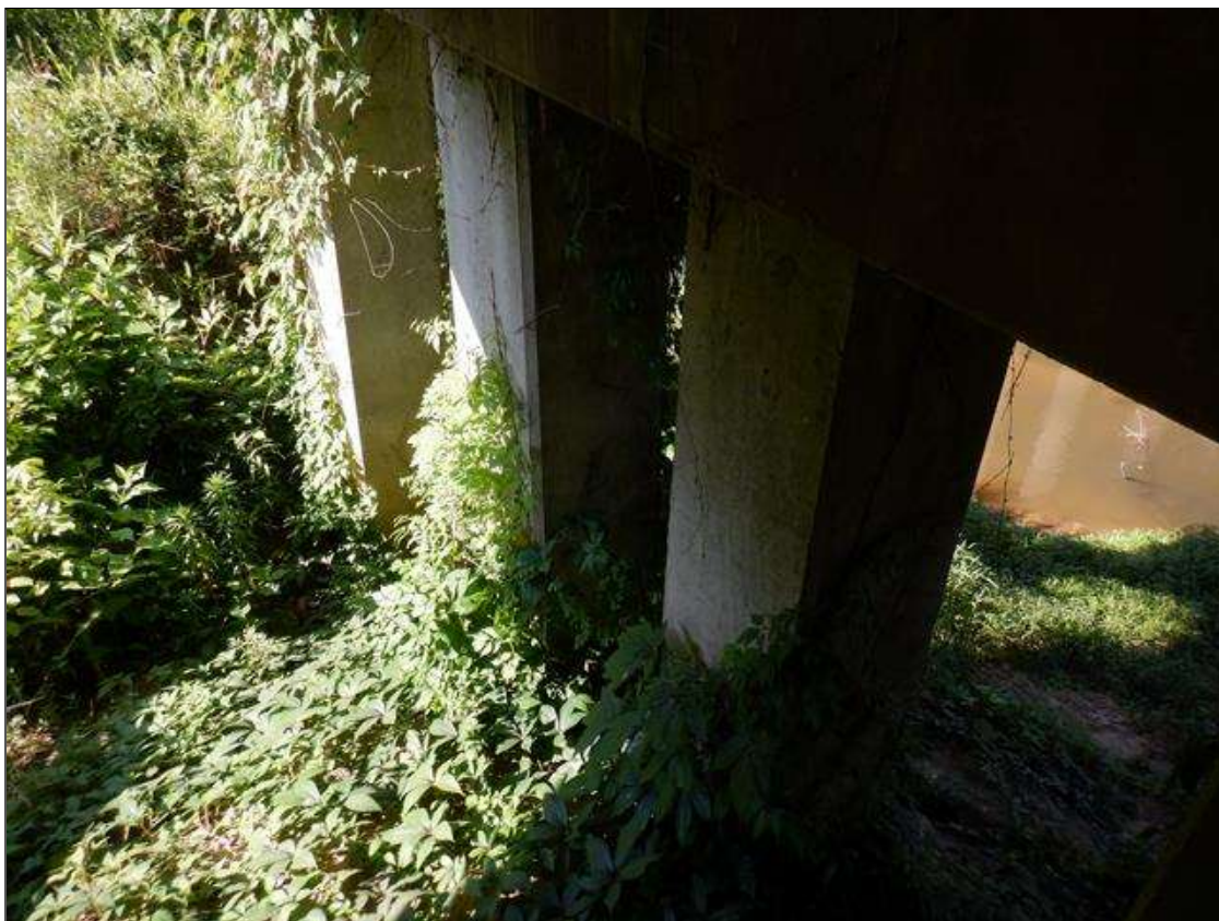
AT BENT 7 VEGETATION GROWTH UP TO FULL HEIGHT ON ALL PILES
